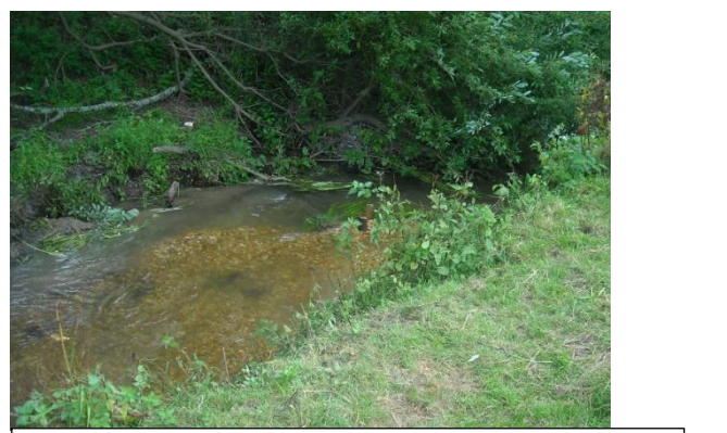
Imported augmented river gravels secured with LWD and improved flow velocity to help self-clean gravels.
