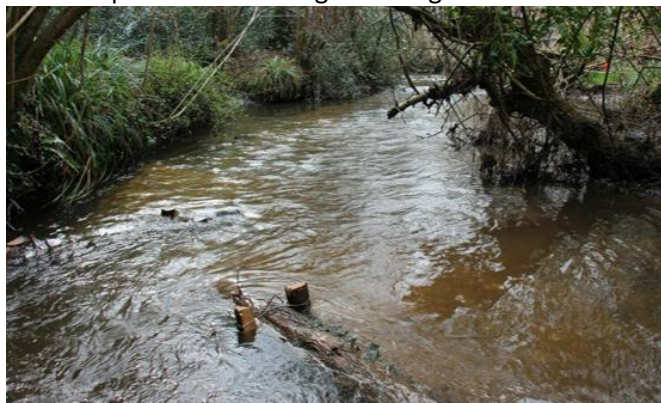
River gravels introduced to a short reach immediately downstream of Burton Mill dam, secured in place with a wooden flow deflector.
